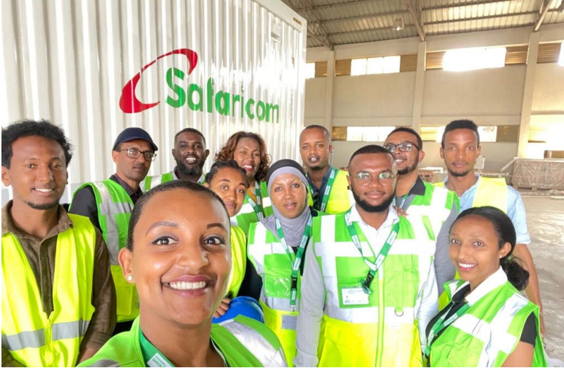
Our Data Center
