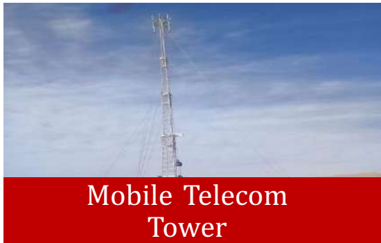
Billboard Structure (Telecom Tower)
