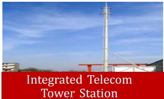
Mobile Telecom Tower
