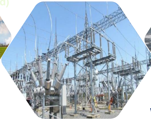
Dedicated Power Substation
