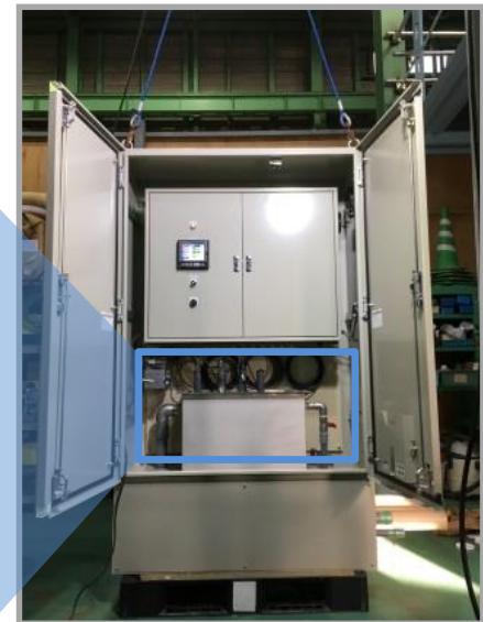
Wastewater Remote Monitoring System in Yangon
