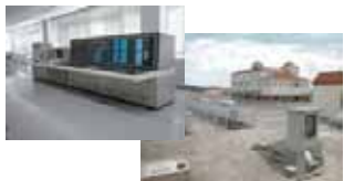
Electric instrumentation systems for water and sewerage
